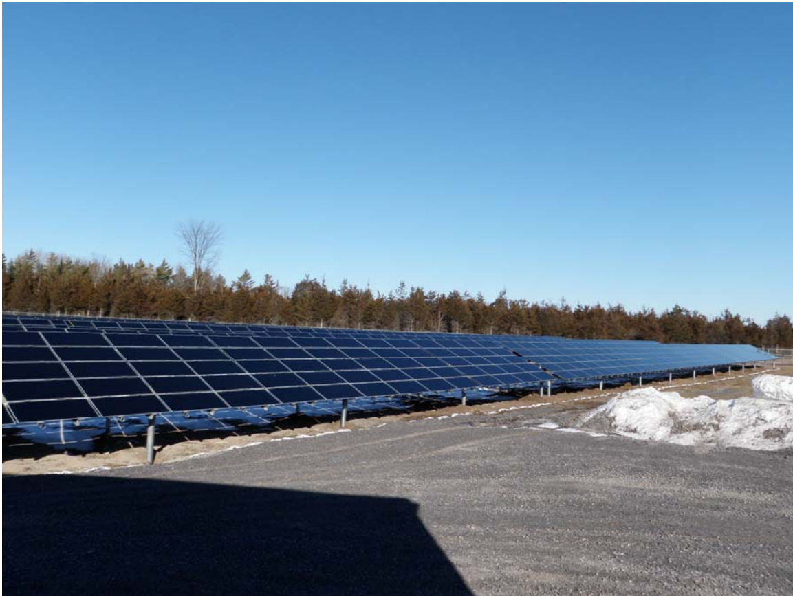
Figure 3.2 Photo of Typical Solar PV Module Installation
