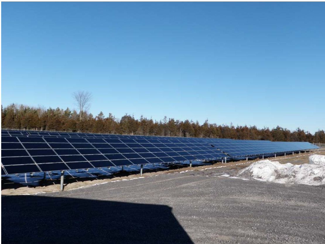
Figure 3.2 Photograph of Typical Solar PV Module Installation
