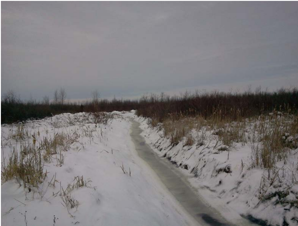
Figure 2.0. Recently cleaned drainage channel through lower Ingleside Swamp PSW north of Project Location (photo taken February 2012).
